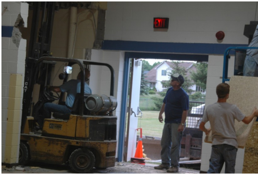
Mike Fedewa and Kurt Thelen remove the ceiling deck of one of the storage closets while Keegan Bengel unloads ceiling tiles.
