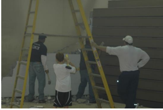
John Miller and Kurt Thelen demolish one of the storage closets while Daric Feldpausch supervises and Tony Hufnagel waits his turn.
