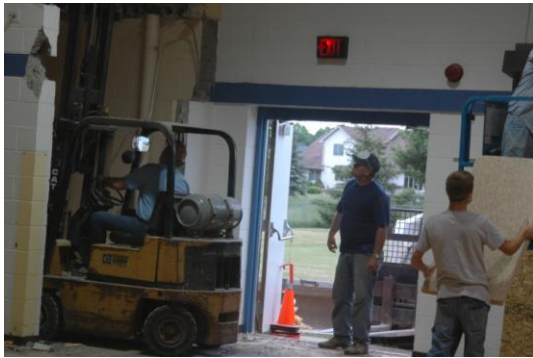
Mike Fedewa and Kurt Thelen remove the ceiling deck of one of the storage closets while Keegan Bengal unloads ceiling tiles.
